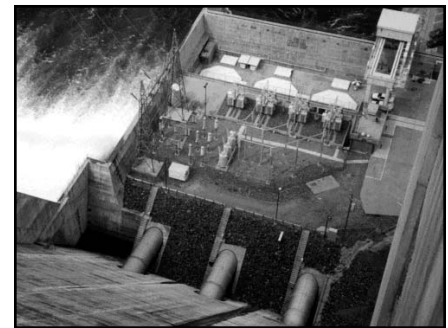
The turbine bypass line will be connected to the power plant's penstocks at the base of Pine Flat Dam.
