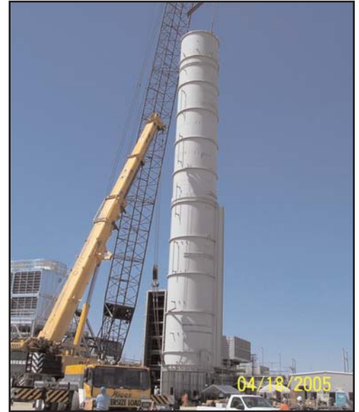
One of two 120 foot tall stacks is erected using one of the largest cranes in the region.
