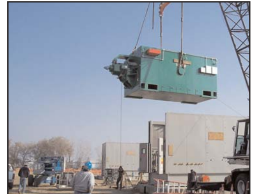
Crews lower one of the generating units into its housing in early December.
